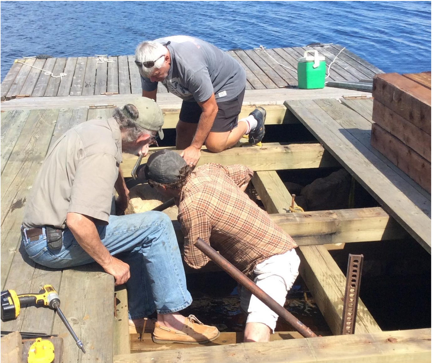
Dock repairs at Goose Lake was a 3-man job! Thank you to Brian for lending a hand.
