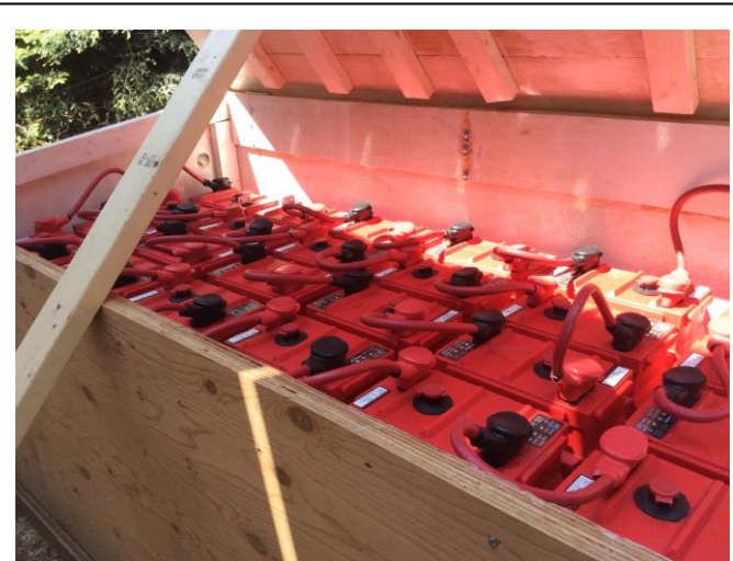
These Surrrette batteries weight 200lbs each and were lowered into the box using the Kubota mini excavator.
